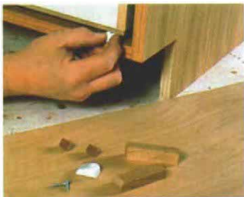
Place guides under the corners of the drawer. A variety of plastic guides are available. The wooden ones are shopmade.
