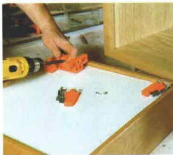
Hidden slides require clips, which go underneath the drawer. The author uses a boring guide from Blum to predrill the mounting holes at the proper angle.
