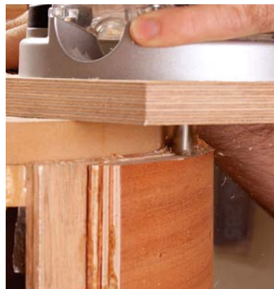
Clean up one edge. With the panel slightly proud of the bending form, a straight bit trims one end square.
