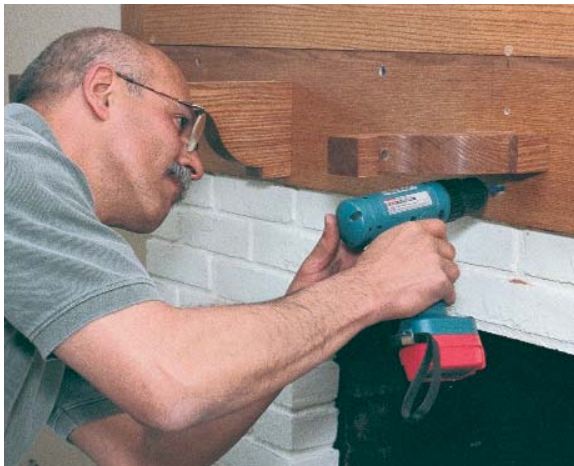
The brackets twist away. When the skirt slides over the brick, the lag bolts allow the author to twist the brackets for easy access to a hidden spot to sink a screw.
