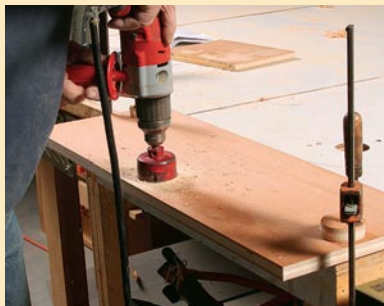
Cut the hole. Casey uses a drill-mounted hole saw, cutting halfway from each direction to avoid damaging the face veneer.
