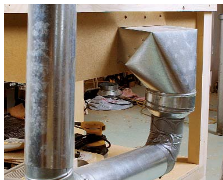
An inexpensive connection. Brown used a standard sheet-metal air-conditioning duct to tie the sanding table to his shop dust system.
