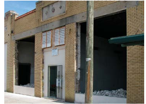
Removing the concrete-block infill and replacing it with glass transformed the space. Once the glass was in, Johnson and Swann installed solar shades made with a mesh fabric that reduces heat gain without blocking the view.
