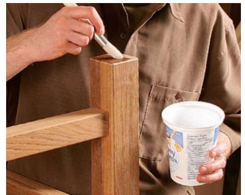
Seal the legs. Seal the bottoms of the legs by coating them with the same epoxy used in the glue-up.
