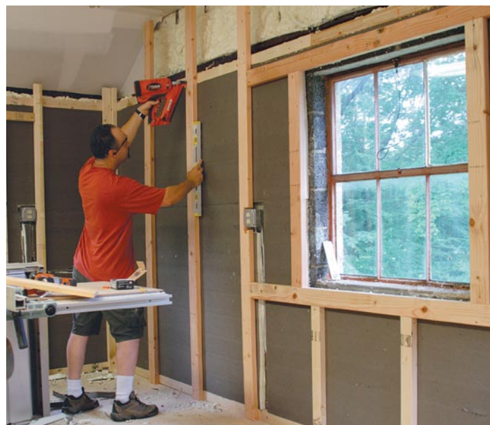
Wall insulation in two layers. With 2x4 nailers already installed top and bottom, the first layer of insulation is put up horizontally and then studs are turned sideways and placed on top. A second layer of insulation is fit between the studs. Use spray foam to seal any gaps between the framing and insulation.
