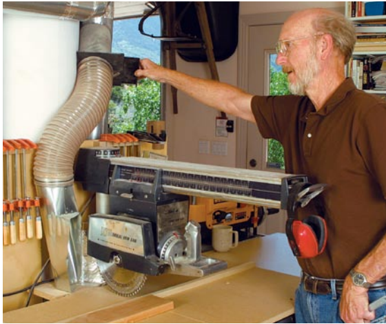
Manual blast gates. Although the dust-collection system comes on automatically when any of the large machines are started, the blast gates are operated manually.
